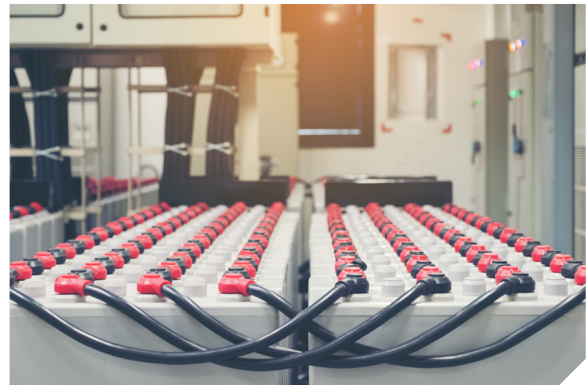
Figure 1. Energy storage battery cells.
