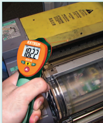
Electrical Troubleshooting for hot spot detection
