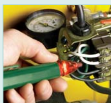
Control panel troubleshooting
