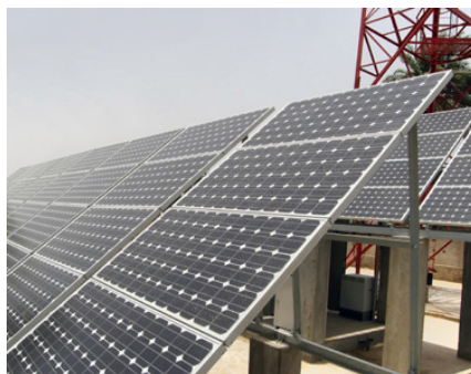
Solar-powered Cellular Base Station
