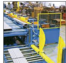
Plant conveying system
